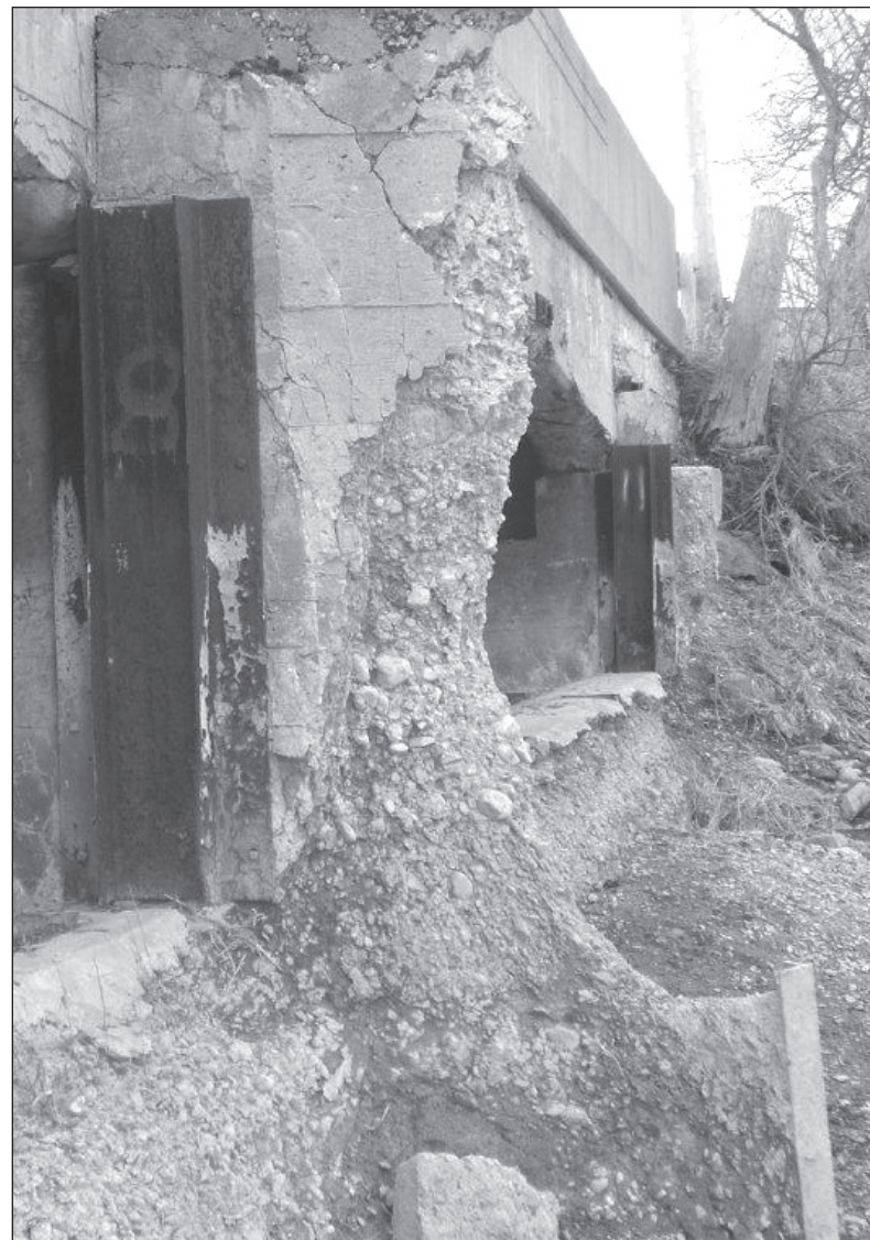
EROSION -Pictured here is a part of the Howson Dam which shows the serious erosion damage, which the entire dam as suffered.
