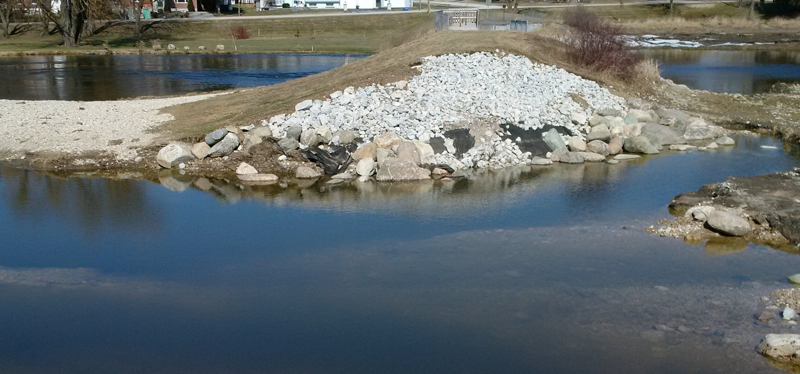
Gorrie Dam failure – June 2017
